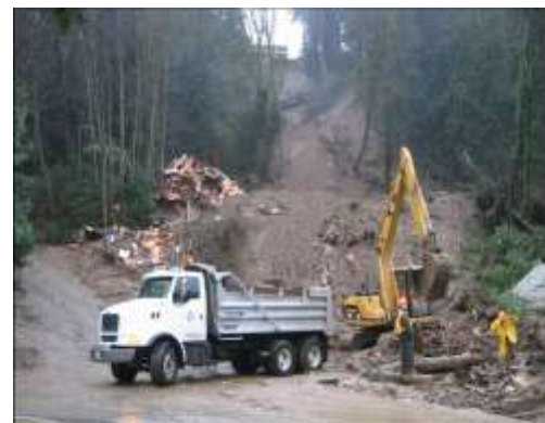
January 2005 flow slide on Berkley Escarpment in the DNV that destroyed a residence and resulted in one fatality.
